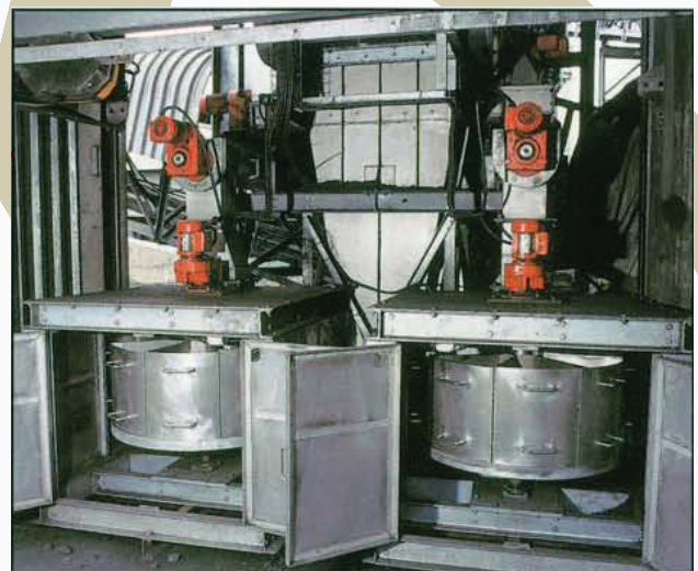
Tertiary cut and final product bins
